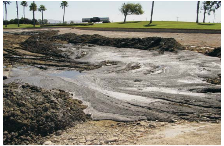
Upon emptying lake, an excessive amount of debris that had collected over the 20 year life of the lake had to be removed.
