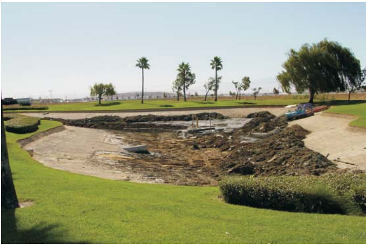
Project: Empty 50,000 decorative lake which was originally lined with a clay/plastic liner. Depth of lake was 15 feet.
