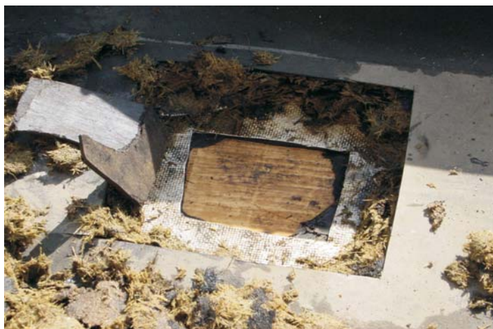
A test cut in the planter box reveals a plywood deck, followed by a 4 ply BUR, followed by a single ply membrane, followed by 1" fiberboard insulation, followed by an EPDM membrane. Insulation is saturated from years of water infiltration.
