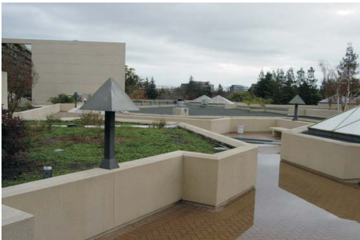
During winter rains, water ponded on the walkways and reports of major leaking into the restaurant and lobby sections required new waterproofing membranes.
