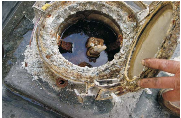
Investigation of the floodlights in the planter section revealed water entering behind corroded o-ring seals.
