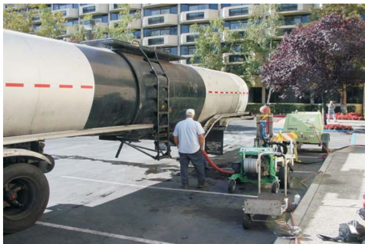
View of a set of doubles containing ~6,000 gallons of The Henry Company's 121 emulsion. Adjacent to the tanker is the WeatherWeld Commander 2021 pumping system, specially developed by the Garlock Equipment Company.
