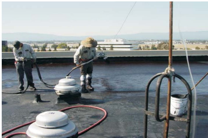
The second application of the WeatherWeld system is being applied on the northern field.
