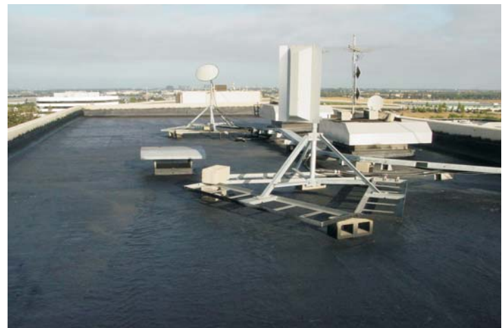
View of microwave antennas mounted on the eastern penthouse of the north roof section.
