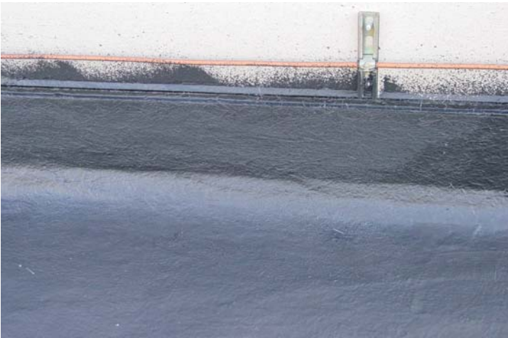
View of seamless composite application from the field, over the baseflashing and up to the reglet of the stucco wall. A new metal counterflashing will be installed after second seamless composite application is completed.
