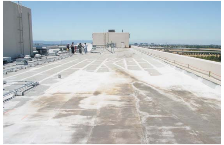
Test cut reveals a structural concrete deck, covered with a tapered insulation system of EPS, covered by ½" fiberboard insulation, covered by a 4 ply BUR set in hot asphalt with a granule capsheet surfacing.
