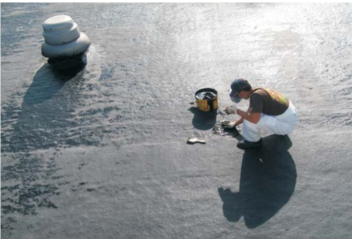
Four random "test cuts" were made to ensure compliance with the manufacturer's specification. Once verified for compliance, the membrane is re-sealed using new seamless composite materials
