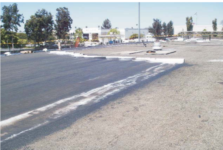
The next operation involves the imbedding of a polyester leveling scrim in 15 gallons of high shear emulsion.
