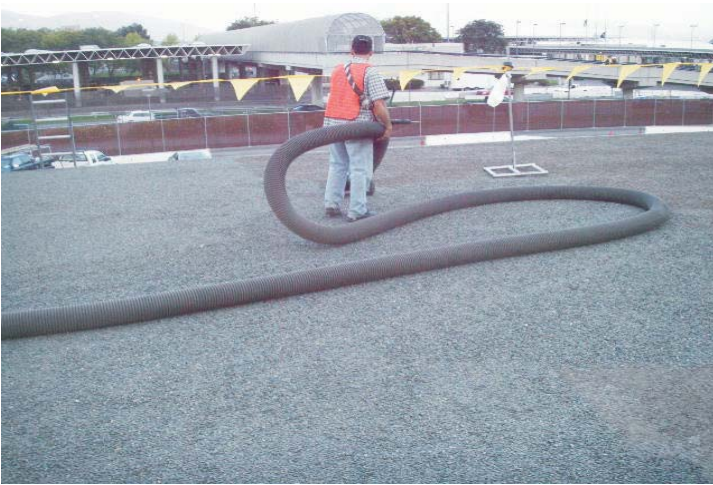
The first step in preparing this roof deck was to vac-broom-vac the loose gravel and embedded dirt.
