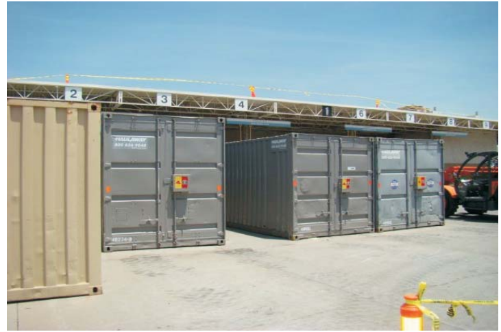
Storage containers with the SunPower PV components are staged on the south side of the Export Building.
