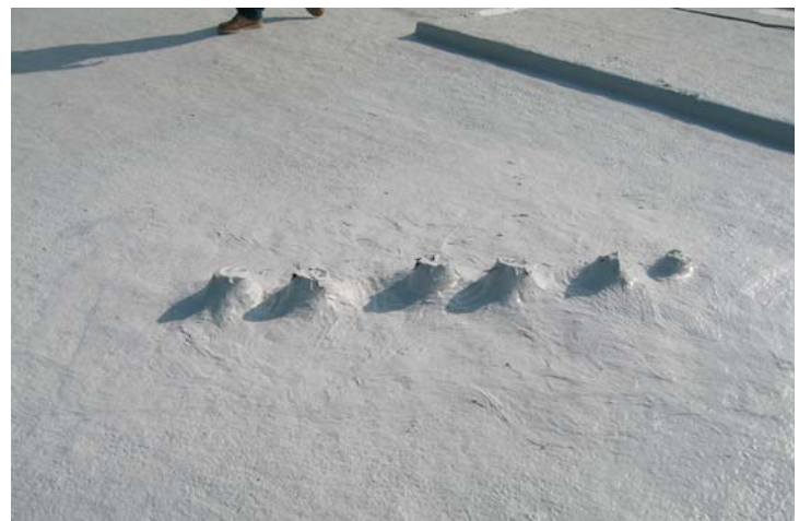
The finished membrane and sealed roof jacks are in place to receive the 274 KW-STC SolarCity solar arrays.
