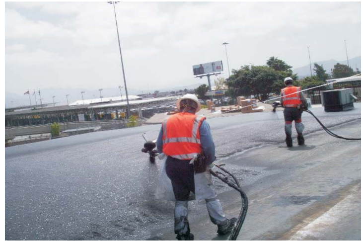
With two applicator guns working together, approximately 25,000 sq feet of roofing can be completed in a single day. The roving and emulsion are combined to form the manufactured-in-place seamless composite membrane.
