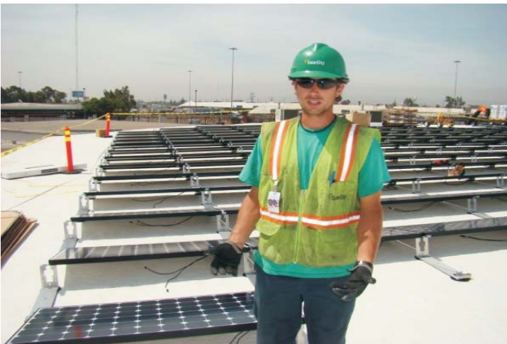
Chris Edgett, Director of Commercial Projects for SolarCity has assigned Jimmy Bergeron to oversee the installation of the PV rooftop elements.
