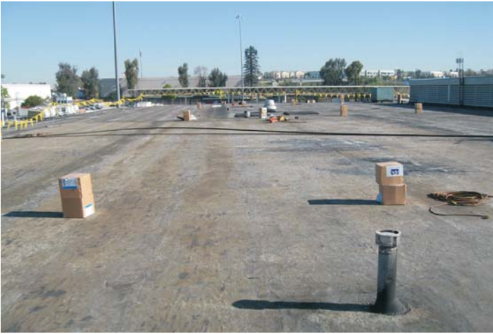
After curing, the prepared surface is now ready for the first of two passes of the WeatherWeld Seamless Composite Materials. Boxes of the fiberglass gun roving are staged on the deck as seen in this photo.
