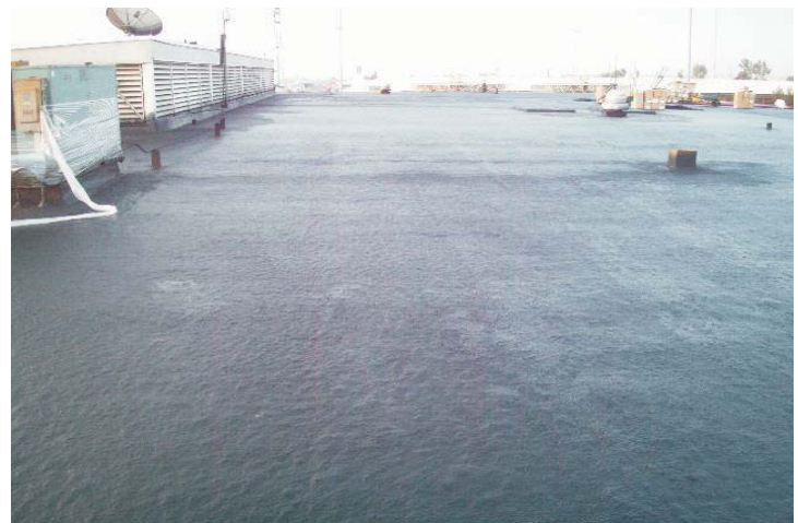
View of the completed 1st pass of the seamless composite materials. Once cured, a second application will be applied.
