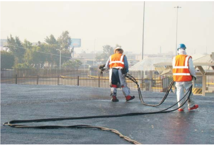
After curing, the WeatherWeld crew applies the 2nd and final pass of the seamless composite materials.
