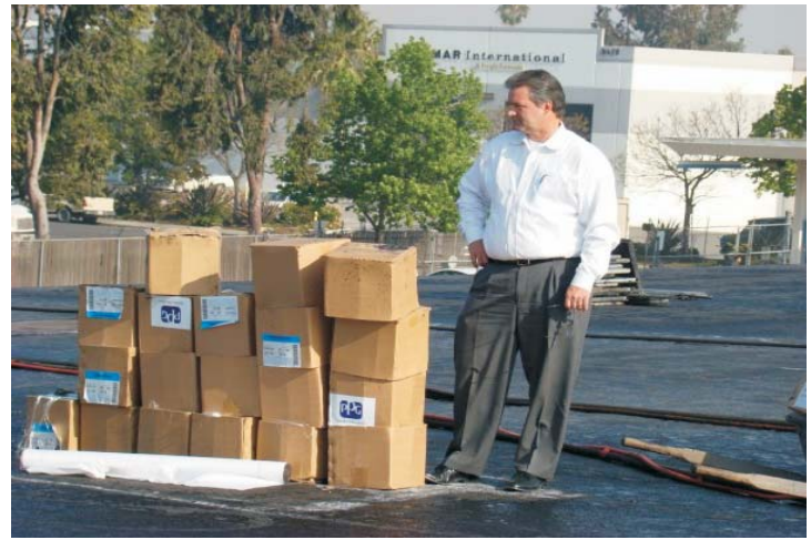
Mr. Tim Cashman, Property Manager for the San Diego Field Office, inspects the progress of the WeatherWeld installation.
