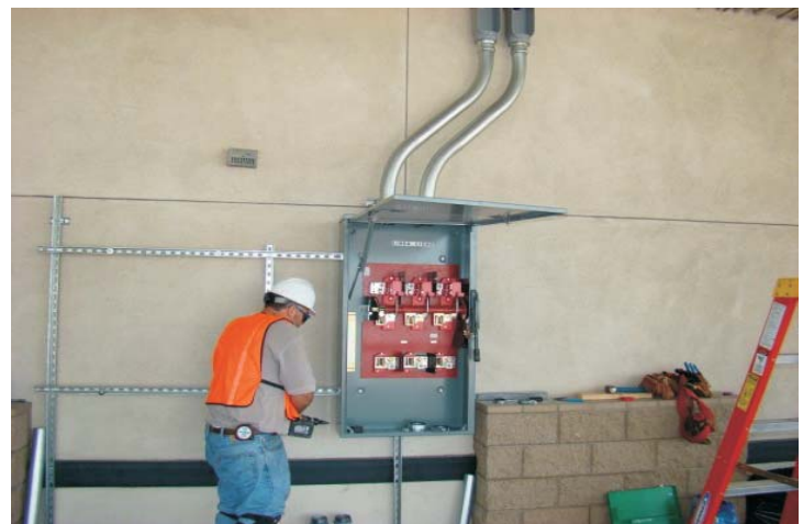
At the SW corner of the dock, a SolarCity electrician is installing the A/C electric disconnect panel.
