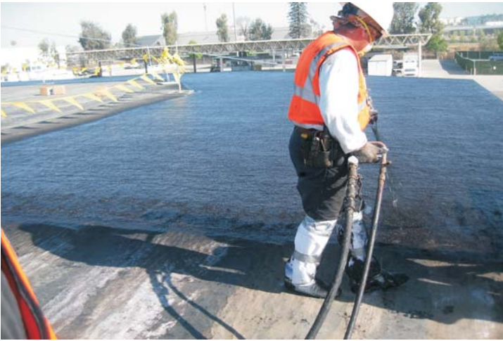
The WeatherWeld crew begins the 1st pass which combines 15 gallons of high shear emulsion with 8 pounds of multi-filament, long strand fiberglass re-inforcement.
