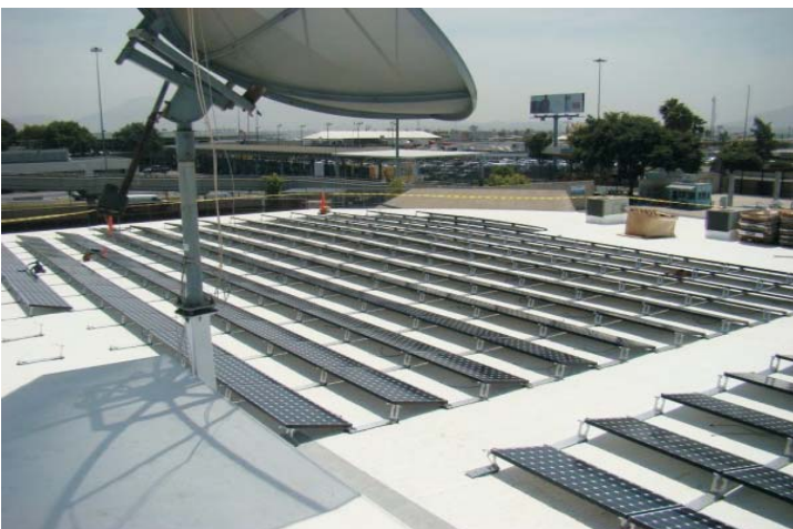
View look SE from the penthouse rooftop. At the end of day 4, approximately 75% of the 1309 Solar Panels had been connected to their rooftop framing members.
