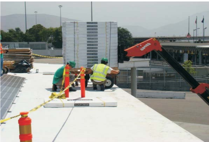
A scissor lift brings a pallet of the SunPower SPR-210 solar panels onto a rooftop dolly.
