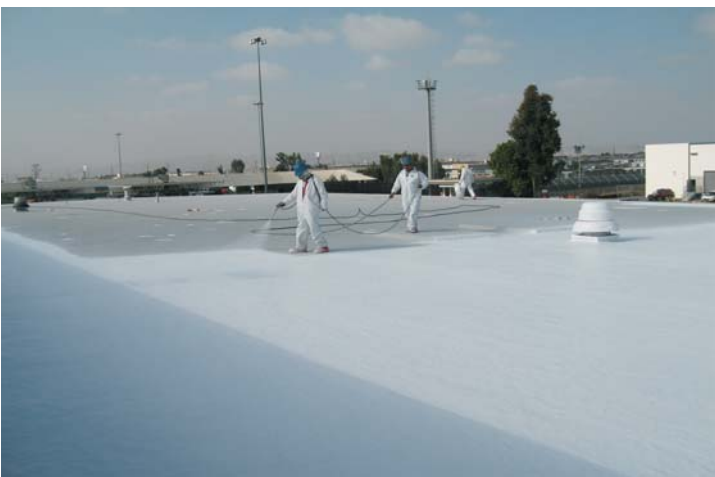
View of the 2nd 1.5 gallon application of lipocryl based reflective coating. The finished WeatherWeld System has a UL Class A fire rating and a 20 year leak proof manufacturer's warranty.
