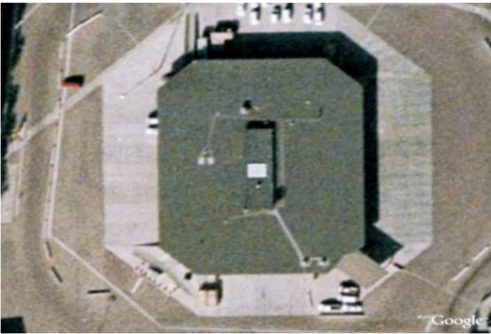
Satellite view of Export Building. A test cut reveals a metal deck, followed by fiberboard insulation, followed by a 4 ply built-up roof set in hot asphalt, followed by a heavy flood coat with an embedded gravel surfacing.
