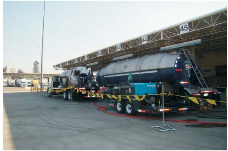
Best Contracting Services stage their equipment on the west side of the facility. It will take over 21,000 gallons of emulsion (four 5,500 gallon tankers) to complete this 46,900 sq foot project.
