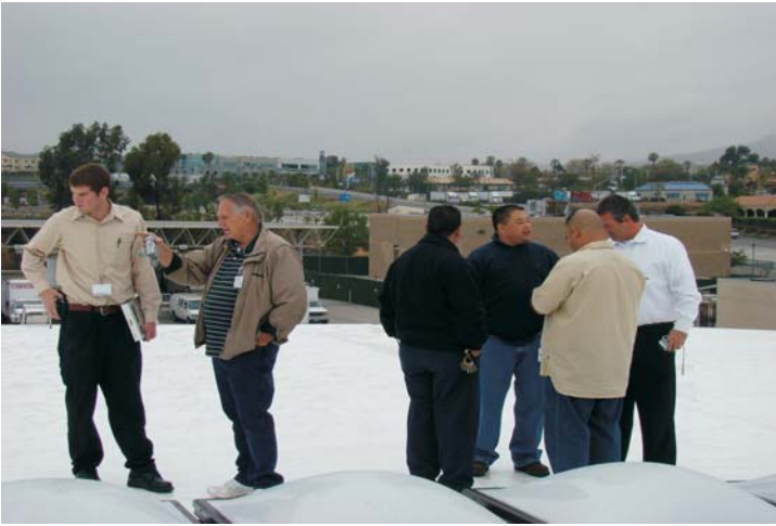
On May 6th, a final walk for the WeatherWeld System was conducted. Present were representatives from the GSA, Hugo Alonso, the GC, Best Contracting Services, and WeatherWeld.
