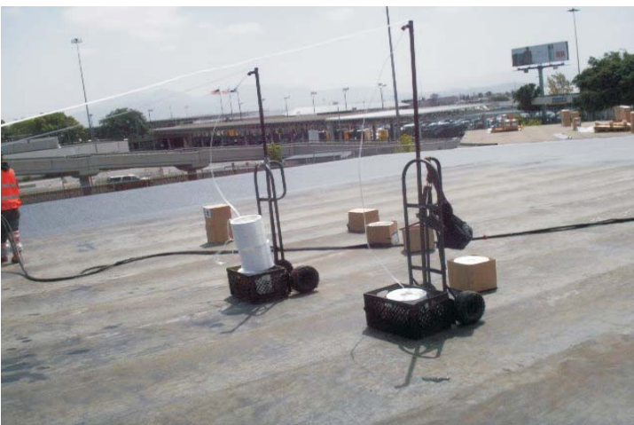
Over 7,500 pounds of fiberglass re-inforcement is being used for this project. The finished WeatherWeld membrane will have over 2.2 miles of fiberglass reinforcement per square foot yet weigh only 1.5 pounds per square foot.
