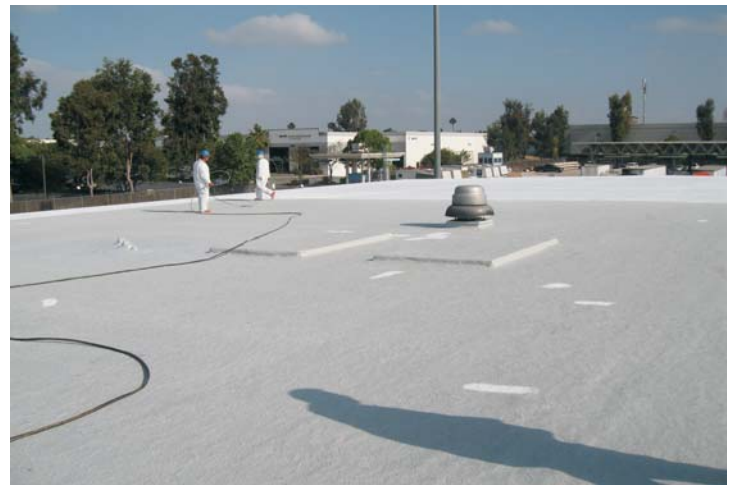
The final operation involves the application of a Title 24 compliant Cool Roof membrane. A 1.5 gallon base coat is applied after the curing of the 2 passes of the WeatherWeld membrane as verified by a Delmhorst moisture meter.
