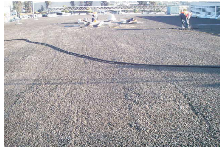
Using this system, an expensive and messy tear-off, impact on landfills, as well as disruptions to normal operations is avoided. This picture shows the prepared roof surface after removal of dirt and gravel.
