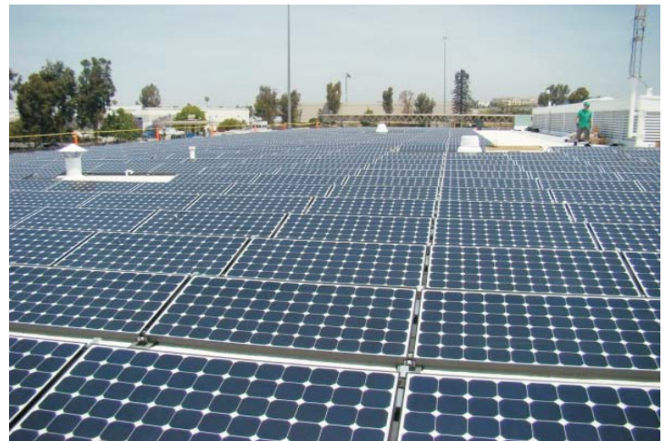
View of low profile panels on the west field of the roof.
