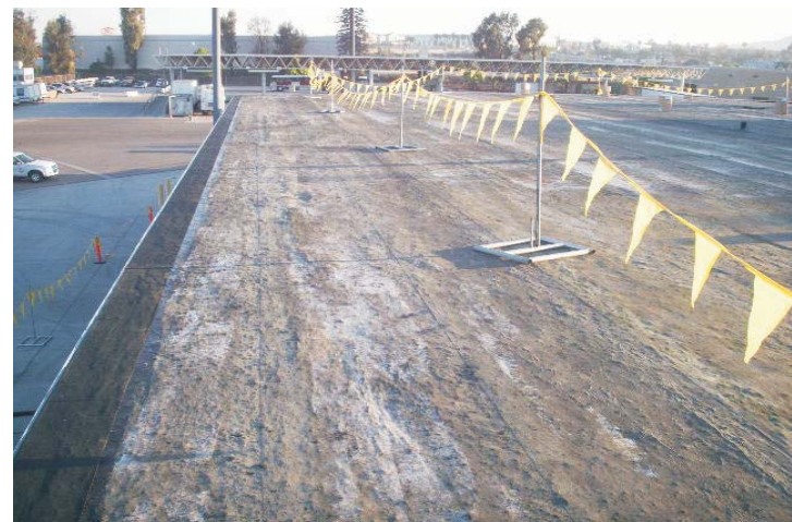
A second generation wide face edge metal was attached to the deck. Next an SBS modified bitumen 75 mil self-adhesive membrane was flashed to the new edge metal and the leveling scrim.
