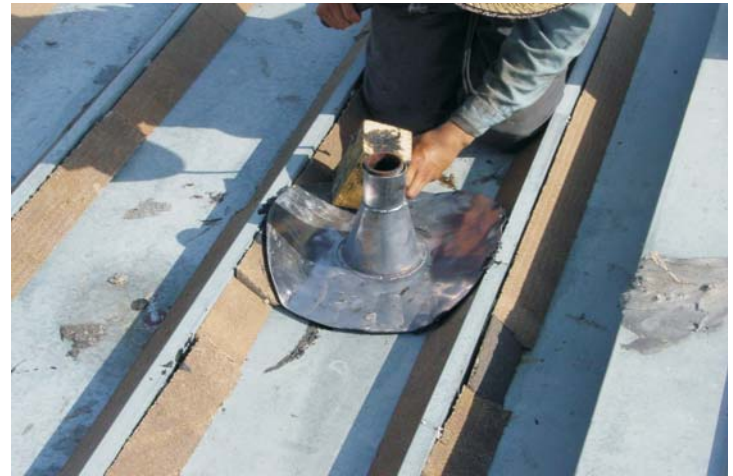
All pipe penetrations are flashed with a lead flashing which is set with mastic and covered with polyester and emulsion.
