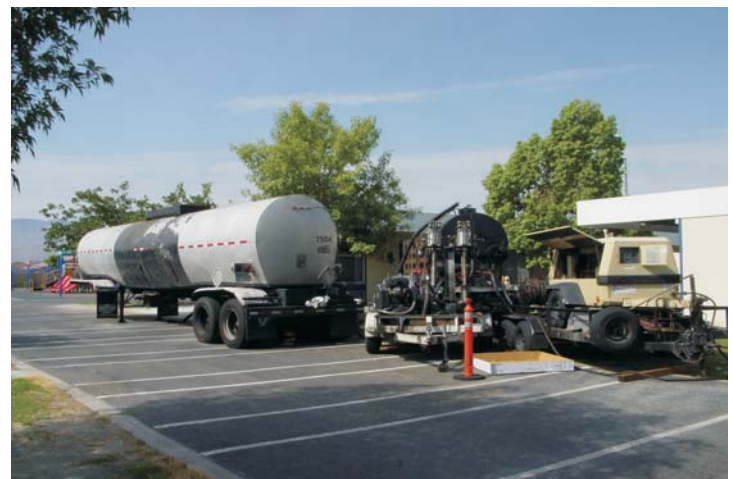
View of staged pneumatic pumping equipment along side a set of doubles containing approximately 6,000 gallons of high shear emulsion.
