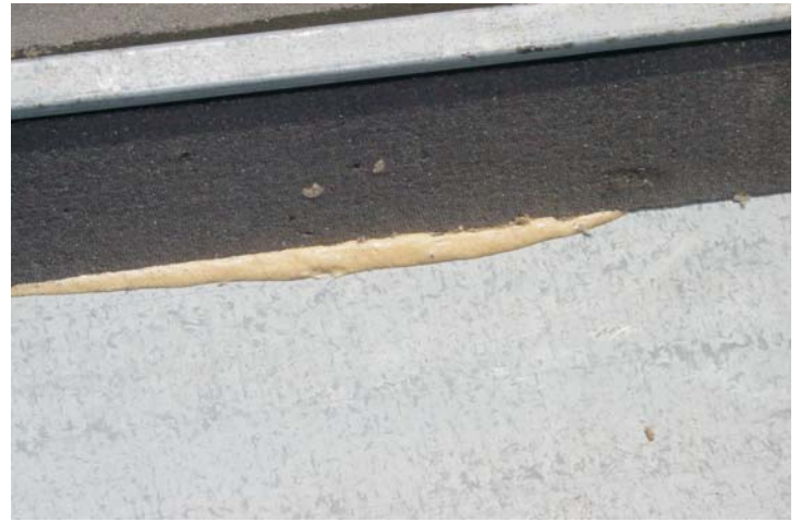
Metal standing-seam panels are power washed. Fasteners are tightened and missing ones replaced. #4 perlite cant strips are set in olybond adhesive against the standing seam.
