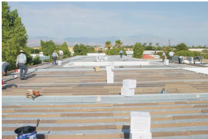
Continuos filament fiberglass roving boxes are set every 6 squares. Each application will have 8 lbs. of fiberglass per square.
