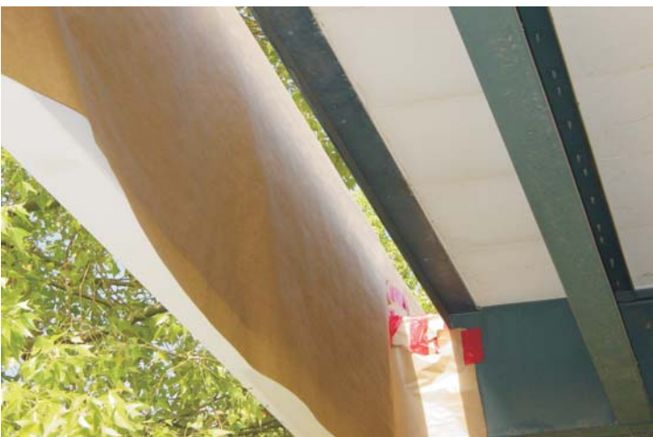
All exposed fascia are covered with masking paper to prevent over-spray on painted surfaces
