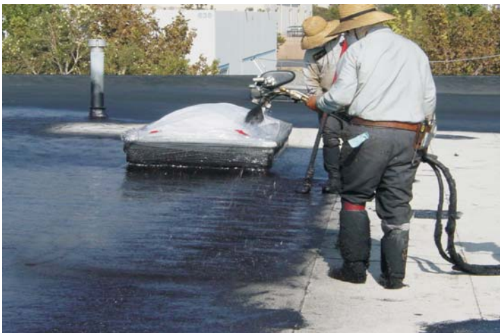
Since a tear-off was not an option, and VOC's, odors and dust were a major concern, the facility's management team selected the WeatherWeld Seamless Composite System.
