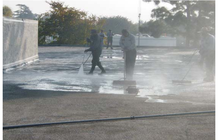
Surface tension is broken. Next, a leveling scrim of 1 ply of polyester is set in 15 gallons of emulsion.
