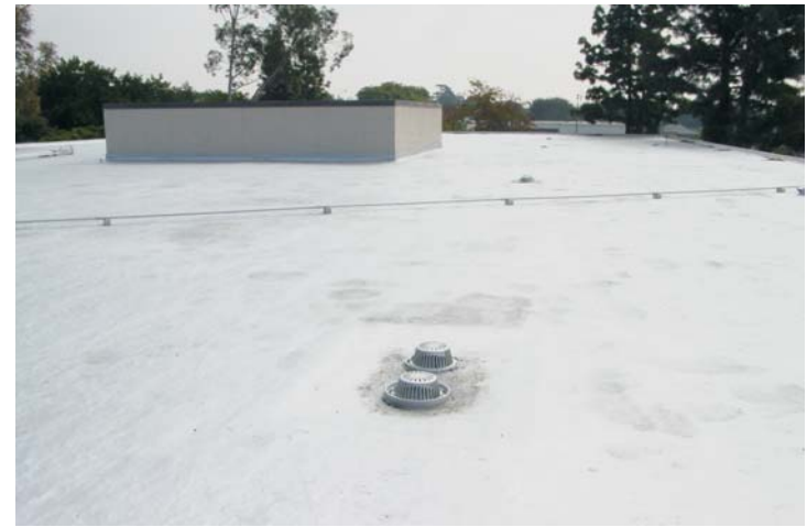
Last, an energy star radiation control coating (RCC) is applied to the finished membrane.
