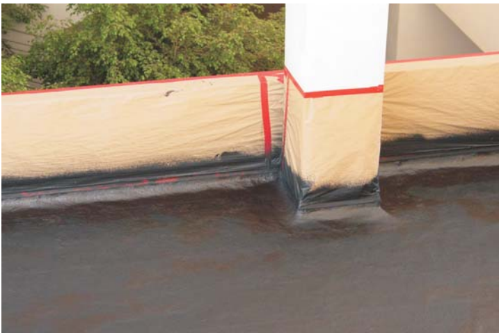
View of western wall of Section "I" showing masking paper covering parapet walls and pillars.
