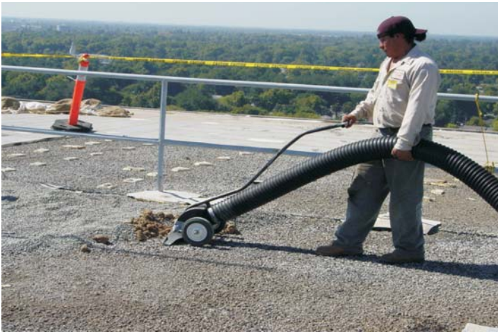
After all the fasteners have been cut, the roof is vacuumed, broomed and vacuumed again.
