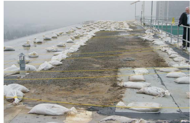
A large rain and wind storm caused a 2,000 square foot section of the PVC membrane to blow-off. The cause of this blow-off was due to wind getting under the southern perimeter metal edging.
