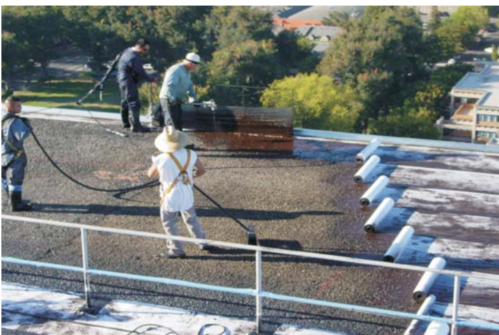
To the cleaned and vacuumed surface, polyester plies are embedded in 15 gallons of emulsion, as a leveling scrim for the WeatherWeld Seamless Composite membrane.
