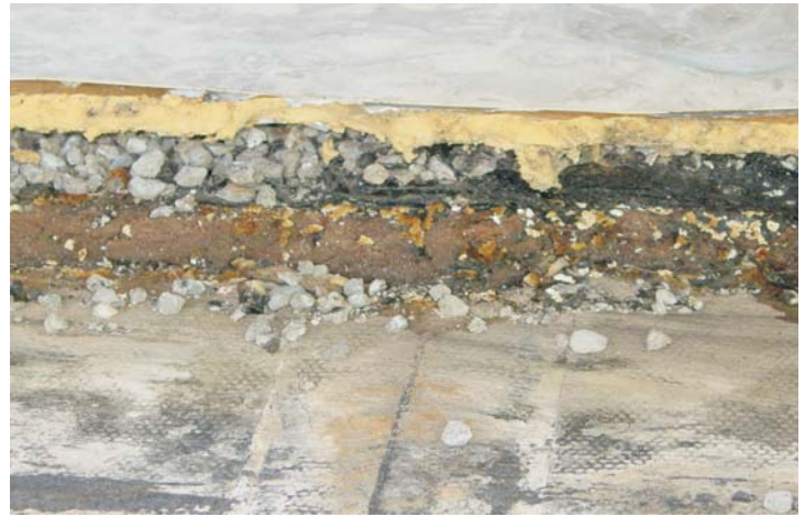
A test cut reveals a steel deck, followed by 1 ½" fiberglass insulation, followed by a 4 ply BUR set in hot asphalt with a gravel surfacing, followed by a recover board, followed by a PC membrane which was mechanically fastened to the deck.
