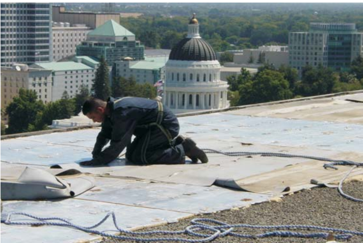
Tear-off involved the removal of the PVC membrane and the recovery board down to the original gravel surfaced roof. There were over 26,000 fasteners attaching the PVC membrane to the metal deck.
