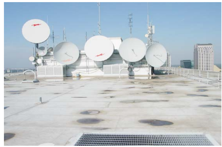
Since there are many critical state agencies resident in this facility, an asbestos abatement was considered unfeasible. The state asked for a work-around practice that could be proposed to waterproof this building without disruptions.
