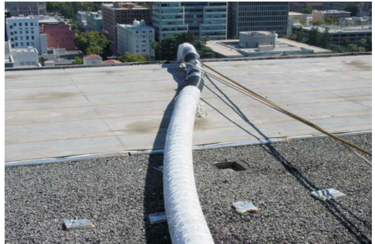
The vacuum hose was tied off at the mid section of the northern perimeter edge.
