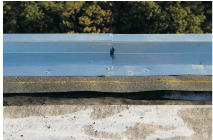
Next came the installation of a new 22 gage metal edging, attached to the original wooden nailer 3" O.C.
