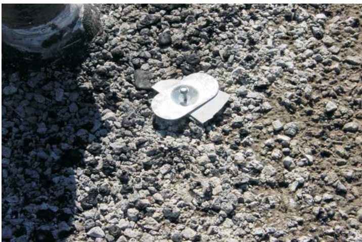
So as not to disturb the fireproofing, a high speed diamond cutting blade was used to cut the fastener at the level of the gravel roof surface.
