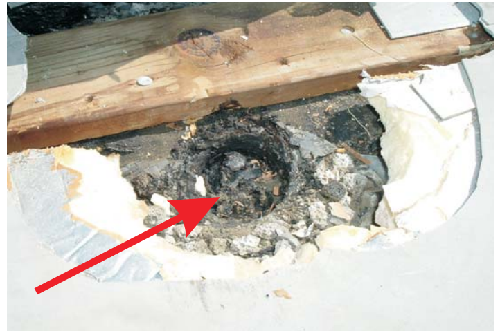
Original 2X6 redwood nailer can be seen at the bottom of this hole. 1x4 wood nailer had to be removed as well as the imbedded gravel for the installation of a new sheet metal edging.
