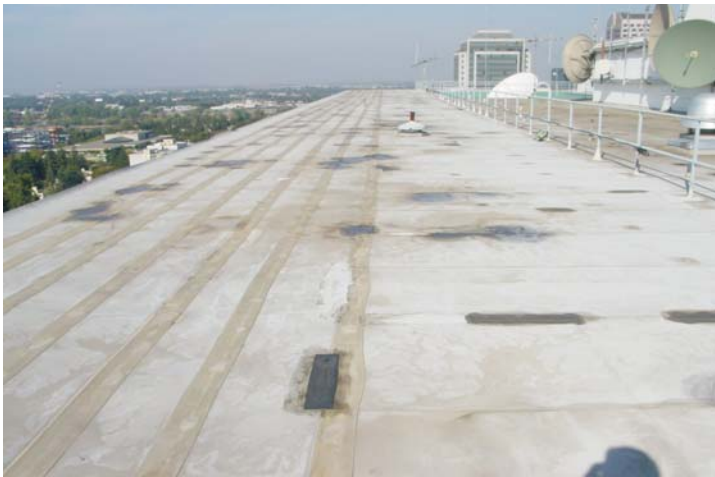
After years of high solar radiation, the plasticizers in the membrane began to bleed out. The membrane then became embrittled and began to shatter as it shrank.
