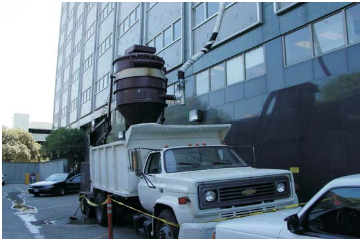
275 feet below, a large vacuum truck collects the gravel to be removed off-site.
