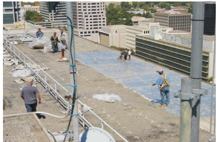
Great care was to be taken so as not to disturb the ACM fireproofing materials on the underside of the deck. The crew is seen collecting the debris in large plastic bags.
