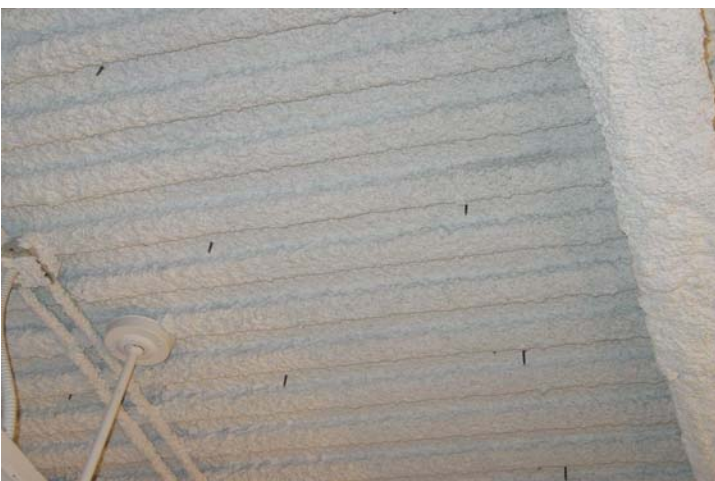
Examination of the lower side of the deck reveals a fire-proofing containing asbestos containing materials.
