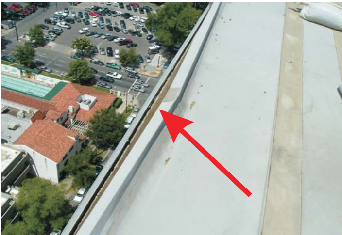
View of perimeter metal edging which failed during the winter storm.
